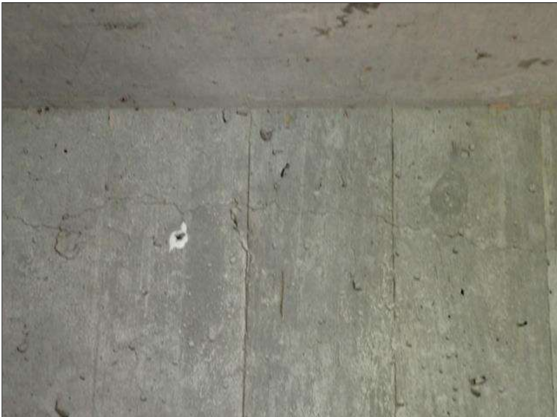
End Bent 1 Abutment: 6' x up to 1/64" horizontal crack WITH EFFLORESCENCE in Bay 3 (Bays 2 and 1 similar)
