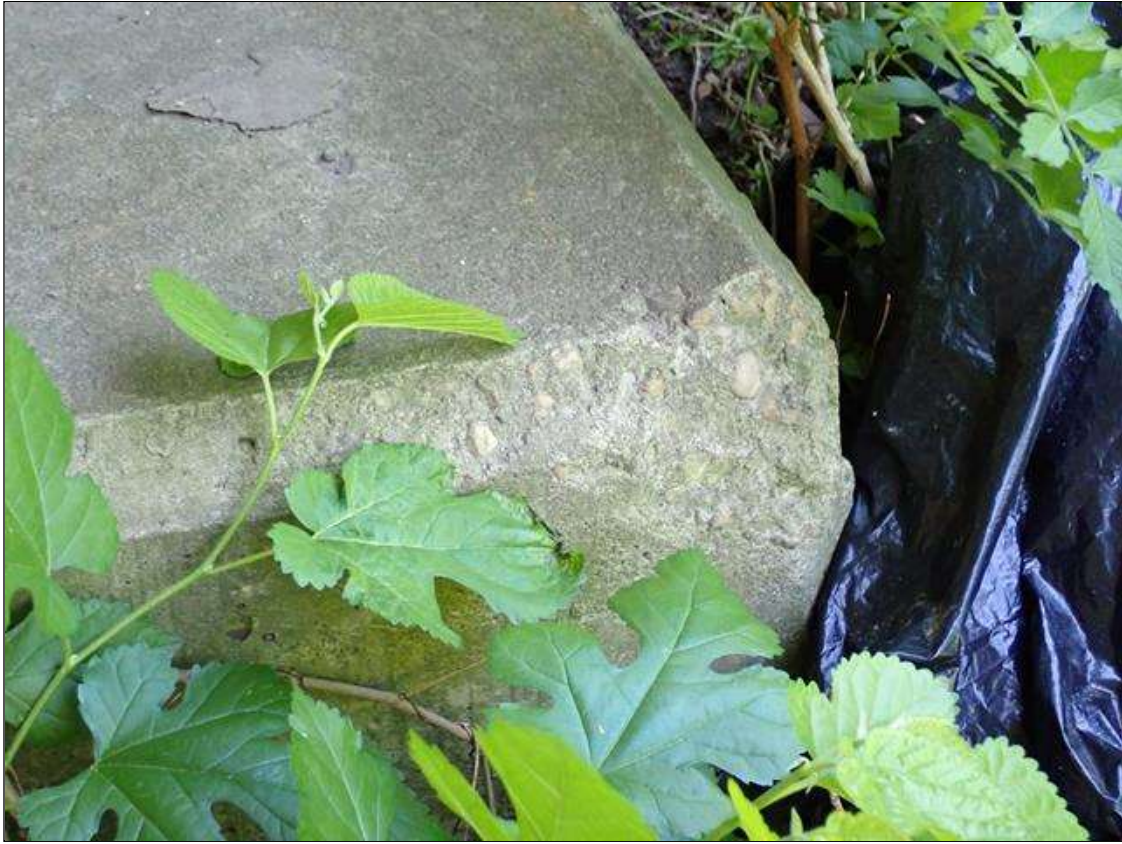
End Bent 1 Cap 1: 4" x 4" x 2" deep spall on Pile Cap 1. No Exposed Rebar.
