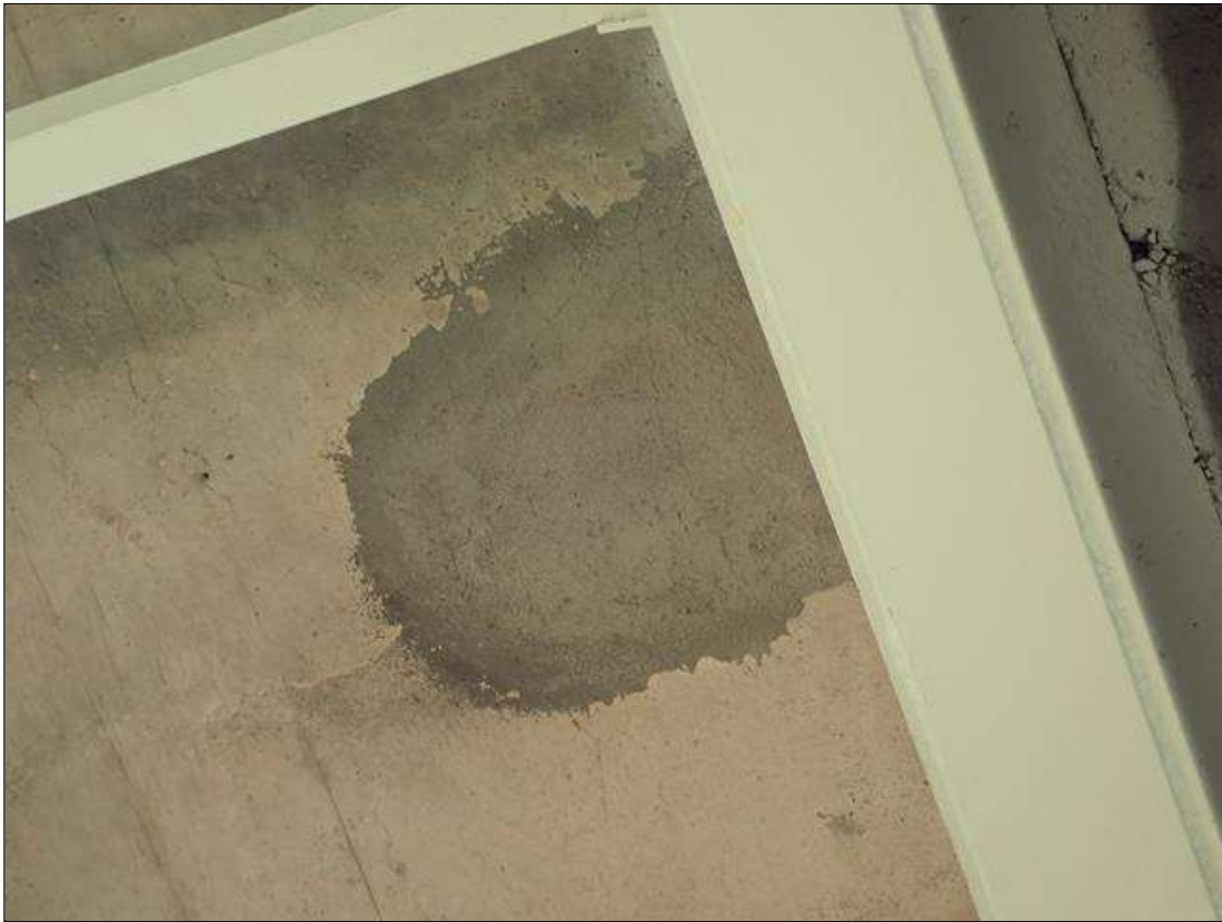
Span 3 Deck: Sound patch 2.5' x 2.5' Bay 3, 16' from Bent 2.
