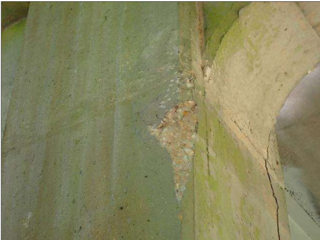
Bent 3 Pile 1: 14" X UP TO 6" X 2" SPALL WITH ADJACENT 1' DIAMETER DELAMINATION ON SOUTHEAST CORNER 2' FROM BOTTOM OF CAP. NO EXPOSED REINFORCEMENT.
