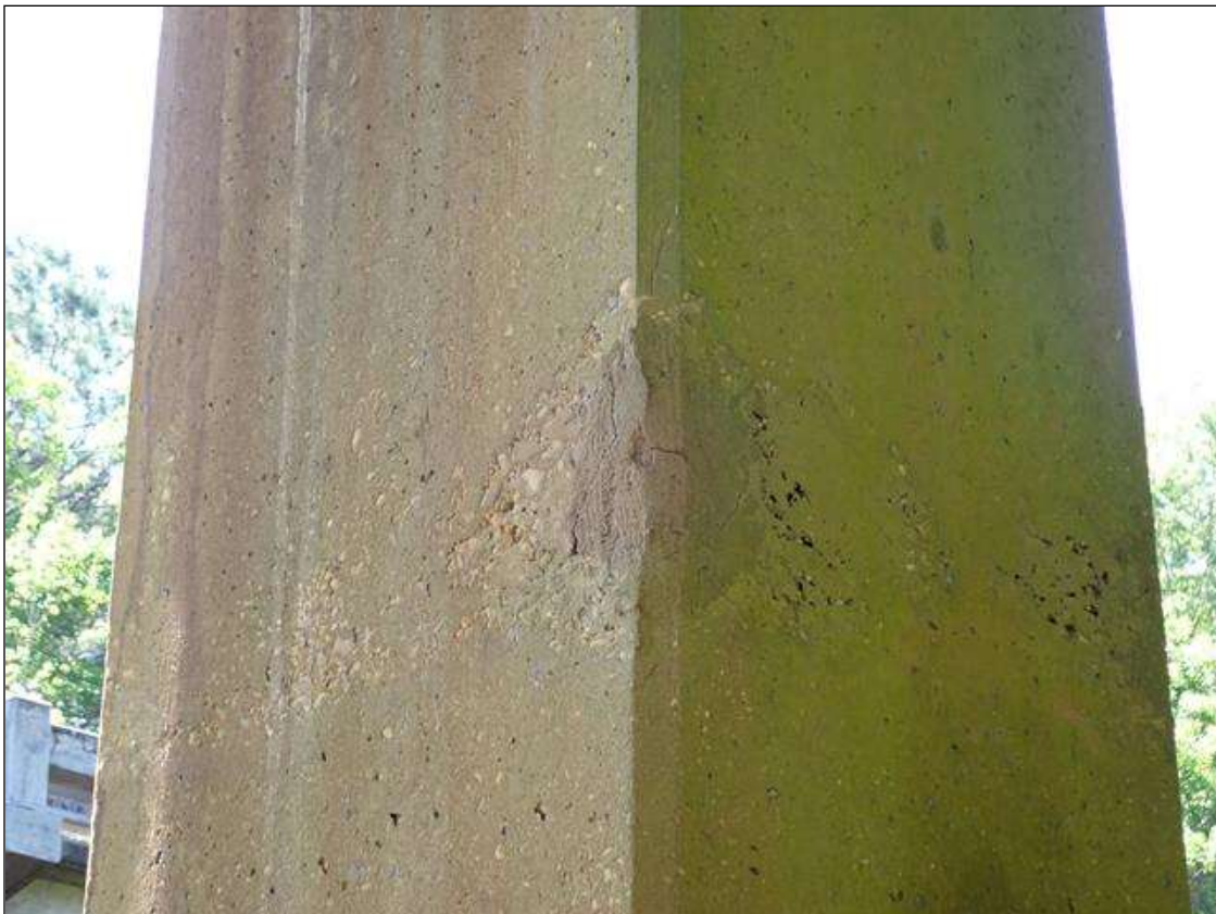
Bent 2 Pile 2: Unsound patch 12" x 8" x 4" North West Corner of Pile 2 below cap.
