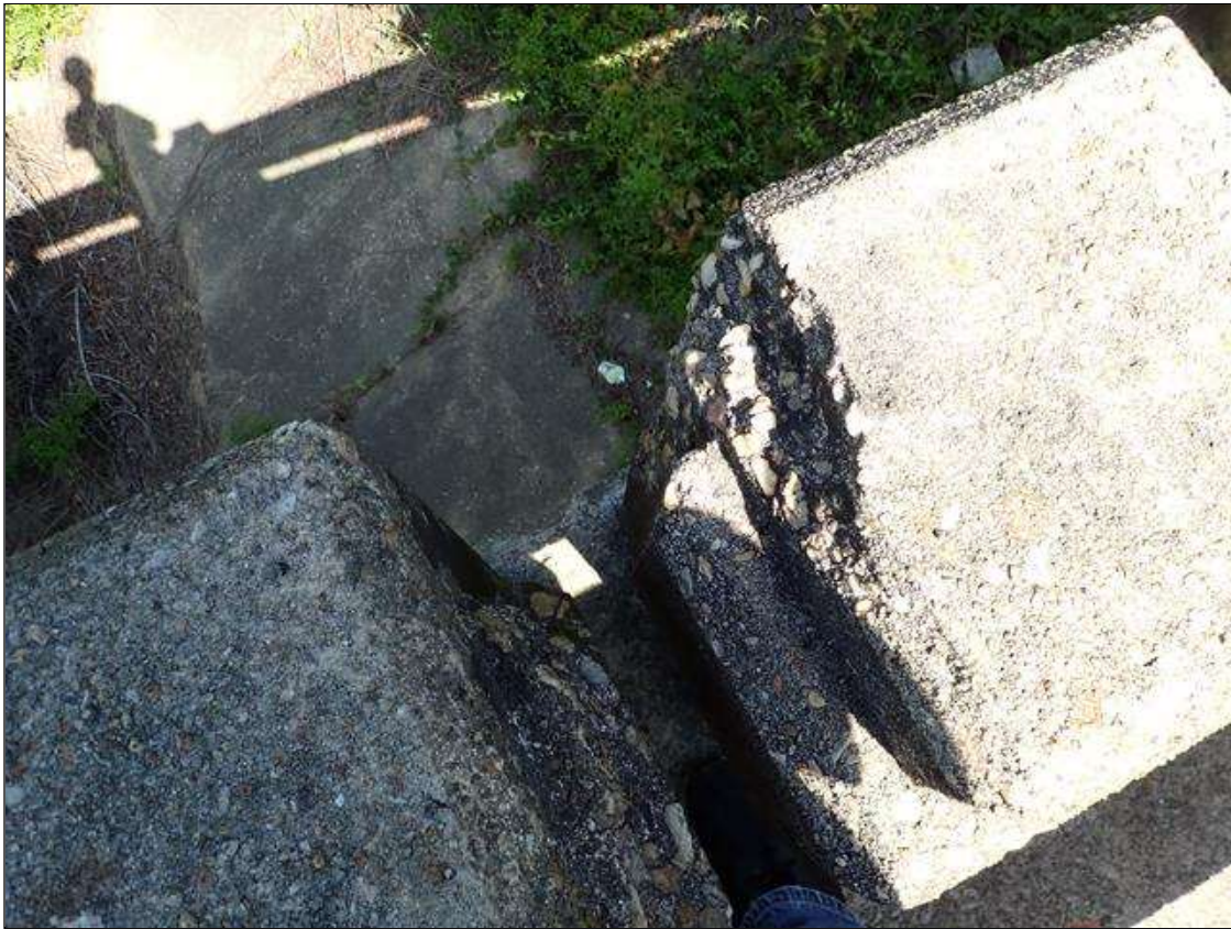
Span 4 Left Bridge Rail: 6" x 1" x 1/2" deep spall with exposed rebar on top of curb, 7' from Bent 3. No measurable section loss.
