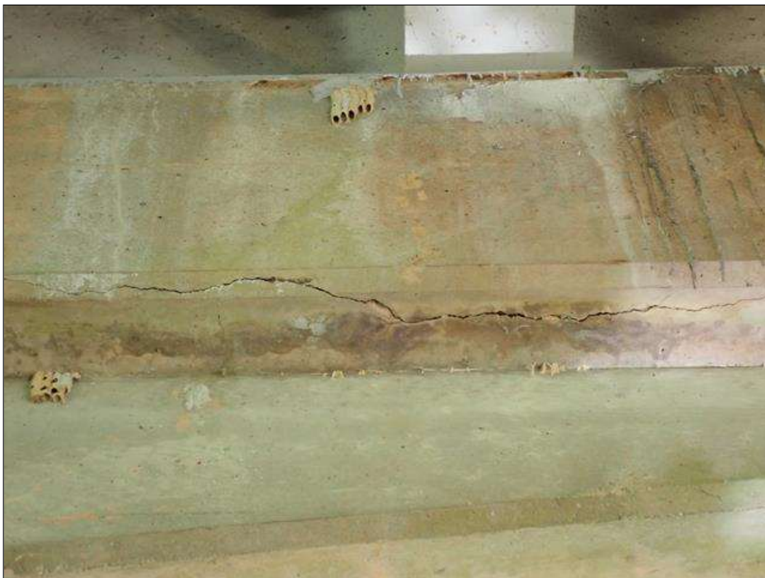
Bent 3 Cap 1: 4' up to 1/8" horizontal crack on Span 3 BOTTOM face UNDER BEAM 2
