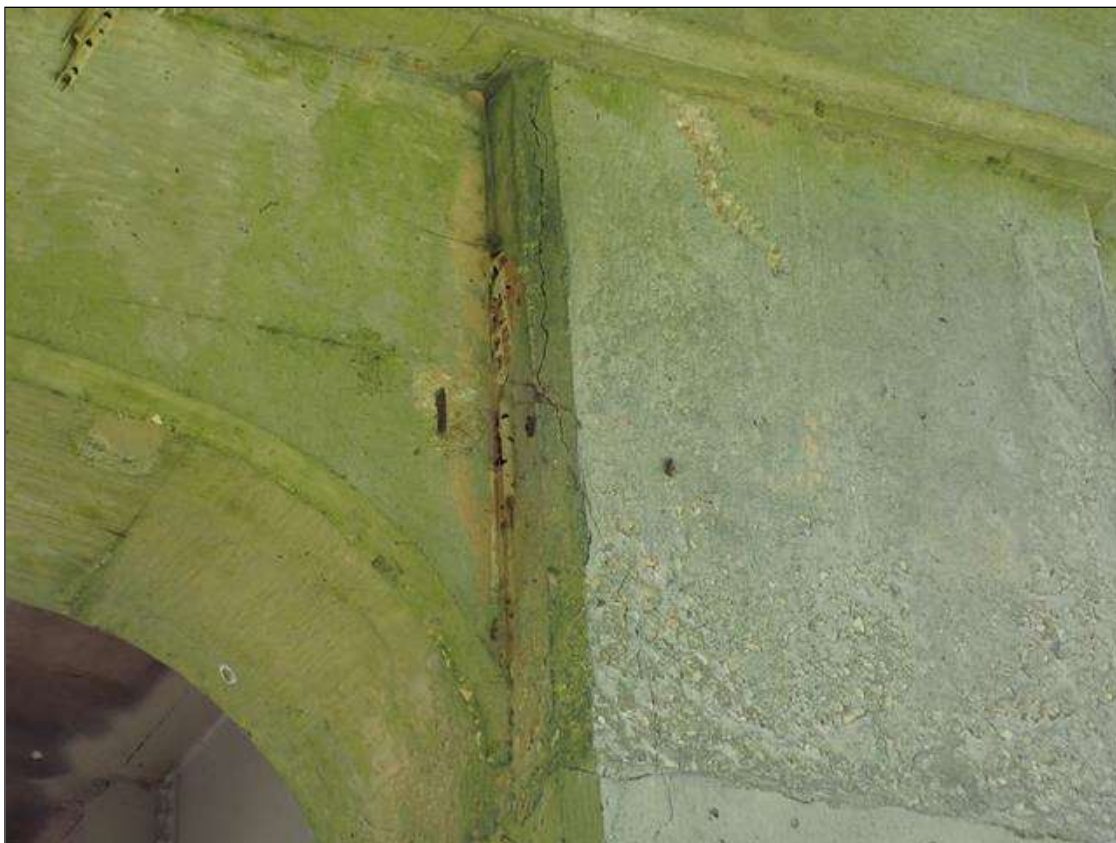
Bent 1 Pile 2: 8" X 2" X 1/4" SPALL AT BOTTOM OF CAP WITH ADJACENT 18" up to 1/16" vertical crack on Span 1 face. No exposed rebar
