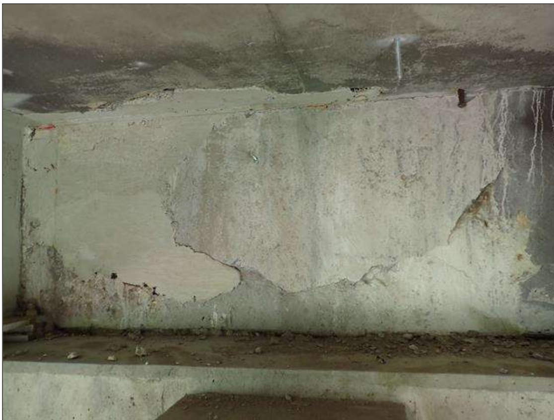
End Bent 2 Abutment: 8' x 2' area of delaminated patch in Bay 2
