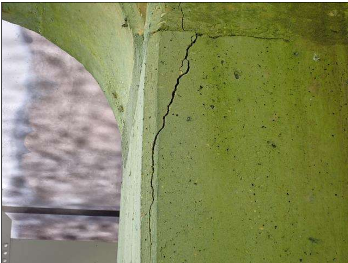
Bent 1 Pile 1: 42" up to 1/4" vertical crack on Span 1 face
