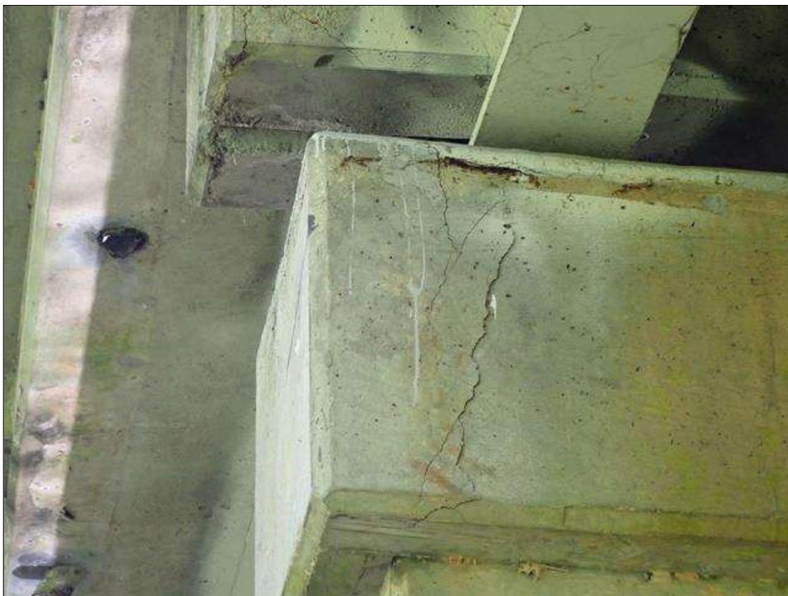
Bent 1 Cap 1: 12" x 24" area of delamination with hairline vertical, diagonal cracks on Span 1 face at West end
