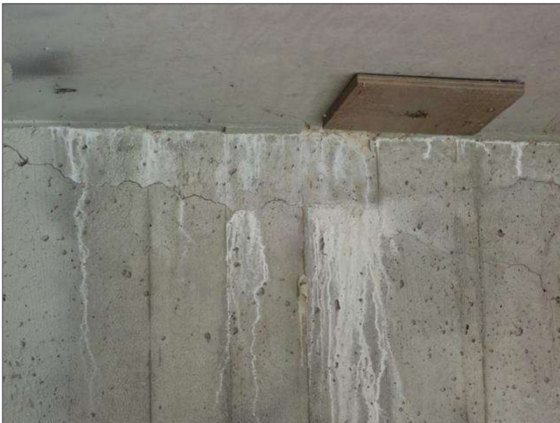
End Bent 2 Abutment: 7' x up to 1/16" horizontal crack with efflorescence in Bay 3
