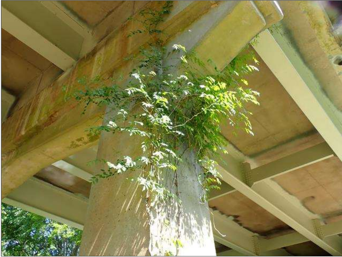
Bent 3 Pile 2: Vegetation around Bent 3 Pile 2.
