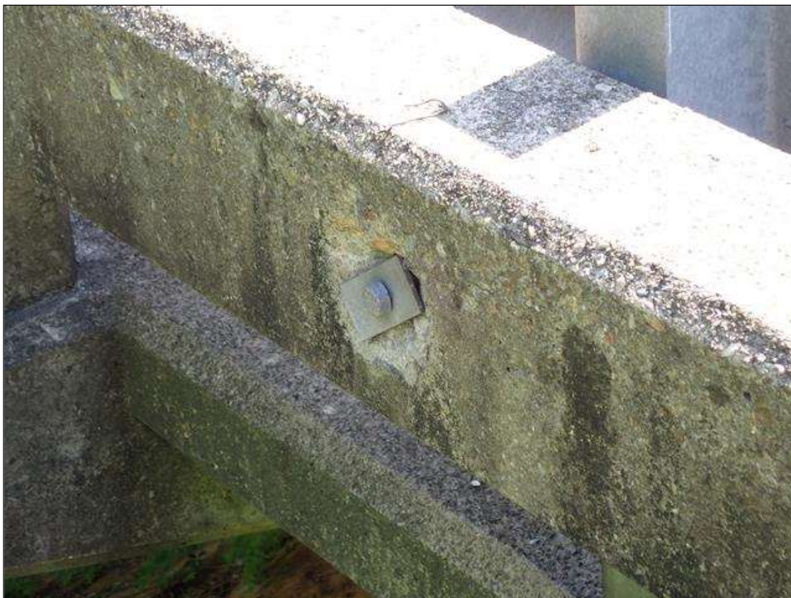
Span 1 Left Bridge Rail: (3) up to 10" x 6" x 1" deep spall on outside face of concrete rail PHOTO TAKEN NEAR END BENT 1. NO EXPOSED REBAR.
