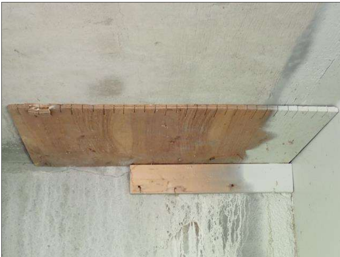
Span 4 Deck: 4' x 2.5' TIMBER STAY IN PLACE FORM WORK IN BAY 1 AT END BENT 2.( 1' X 1' SIMILAR IN BAY 3)
