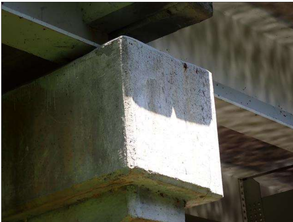
Bent 1 Cap 1: Unsound patch east end of cap. Full height x Full width x 1' long cracking.
