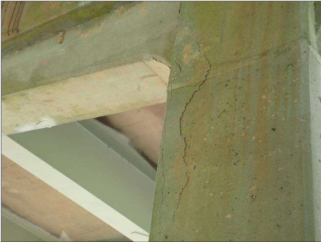
Bent 3 Pile 1: 4' x 1' x 8" delamination at north east corner of pile 1, 2' below cap.
