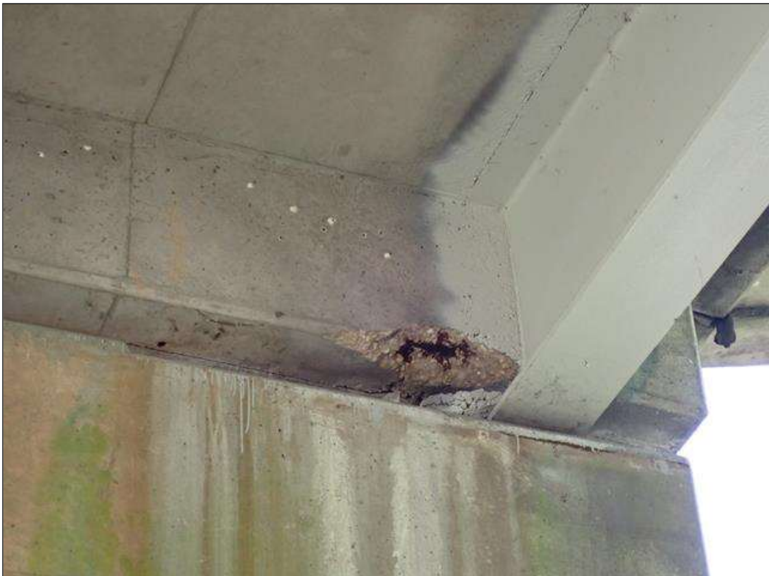
Span 4 Beam 1 end diaphragm at bent 3, bay 1 with a spall, 2 ft x 6" x 6" with exposed rebar, no measurable section loss adjacent to beam 1
