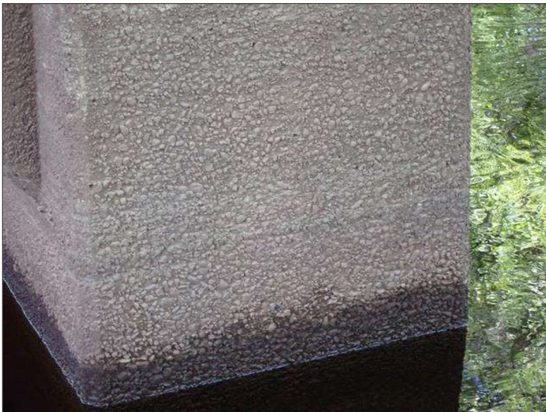
Bent 2 Pile 1: 4' ABRASION/WEAR 15' FROM BOTTOM OF CAP. AGGREGATE INTACT
