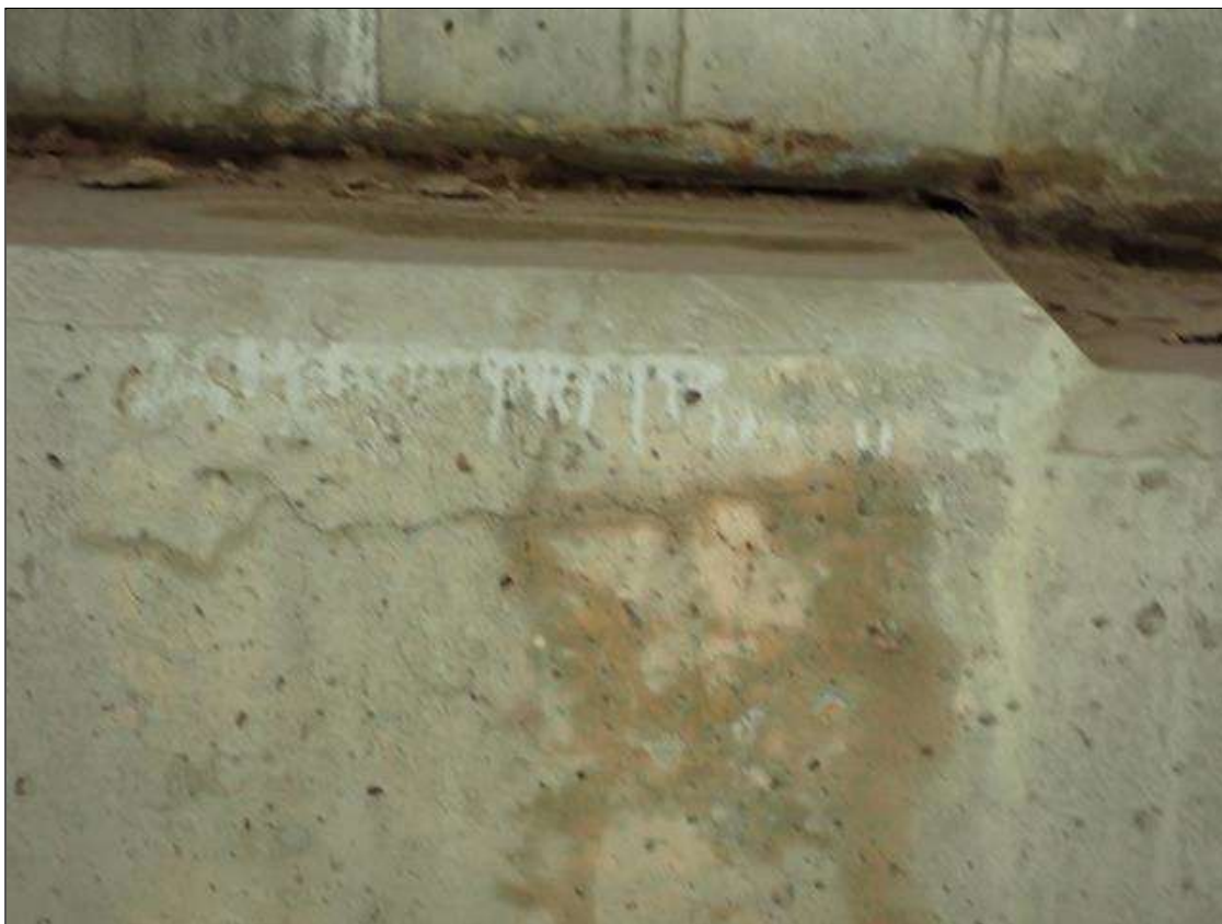
End Bent 2 Cap 1: 15" x up to 1/64" horizontal crack under Bay 3
