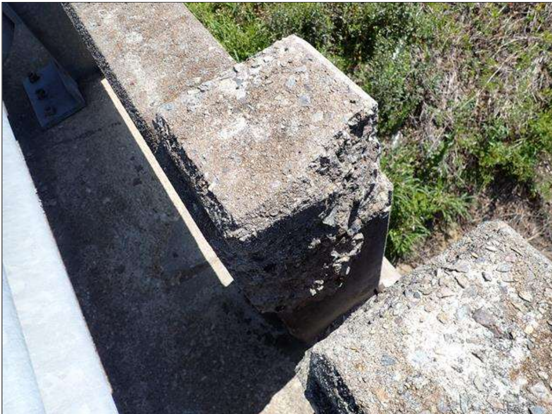
Span 4 Right Bridge Rail: 2" x 8" x 10" deep spall with exposed rebar on concrete Post 7 (Post 6 similar) no measurable section loss
