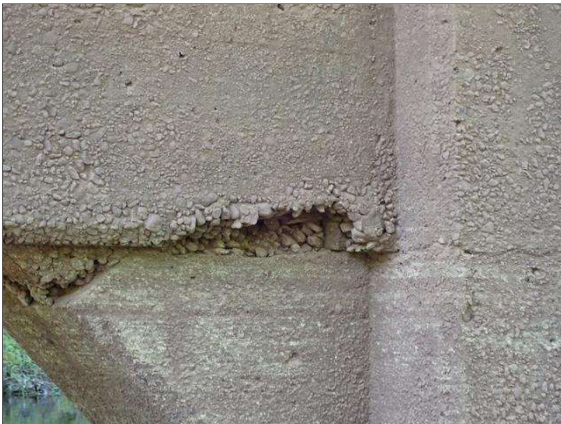
Bent 2 Pile 1: 10" x 2" x 2" deep spall on Span 3 face of strut. No exposed rebar.
