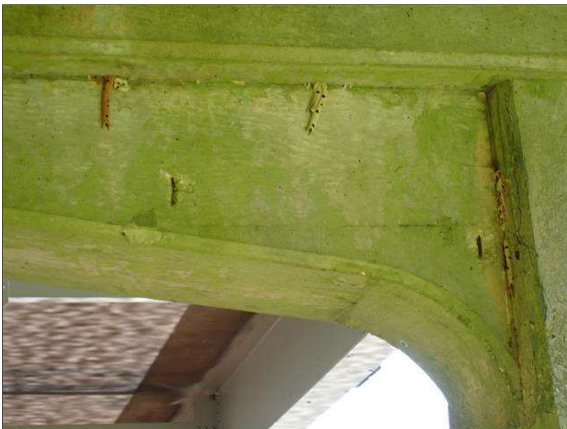
Bent 1 Cap 1: (2) up to 3" x 3" x 1" deep spall with exposed rebar on corbel on Span 1 face no measurable section loss
