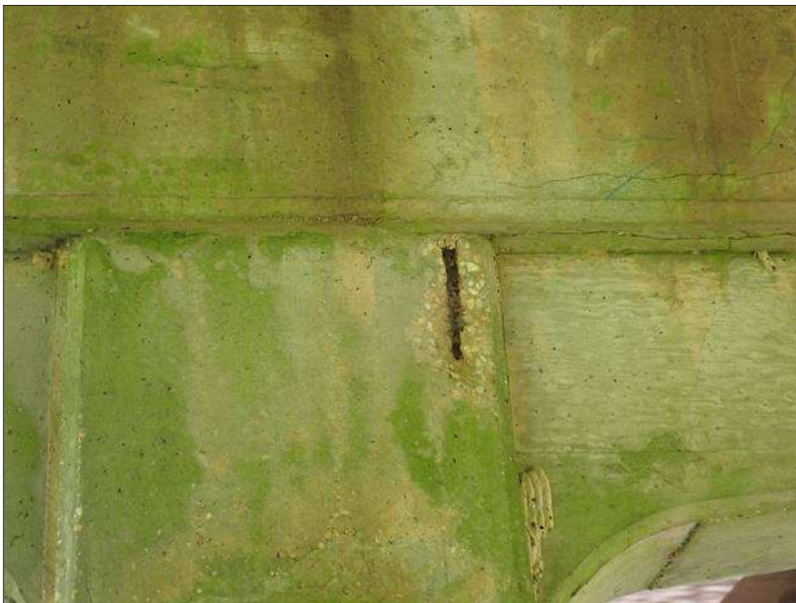
Bent 1 Pile 1: 12" x 5" x 1" SPALL WITH EXPOSED REBAR ON SOUTH FACE AT BOTTOM OF CAP. NO MEASURABLE SECTION LOSS.
