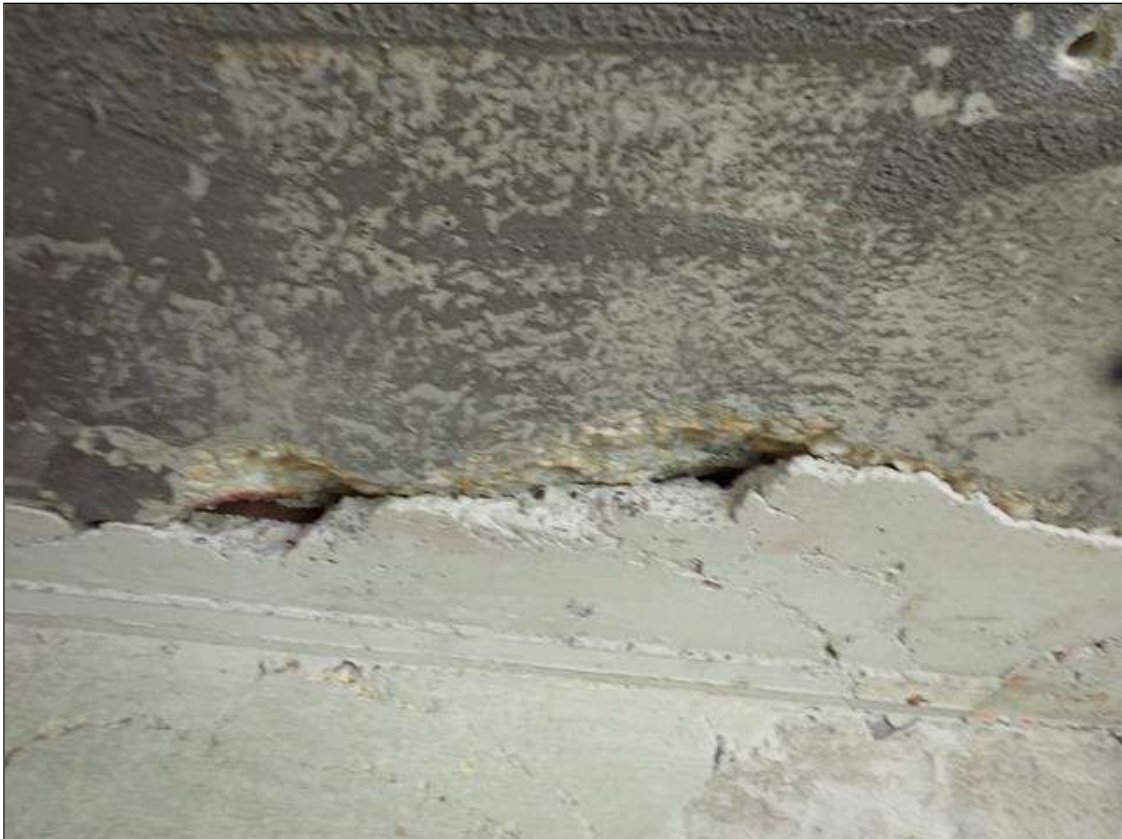
Span 4 Deck: Spall 17" x 4" x 2" deep in underside of deck in bay 2 at end bent 2 with no measurable section loss.
